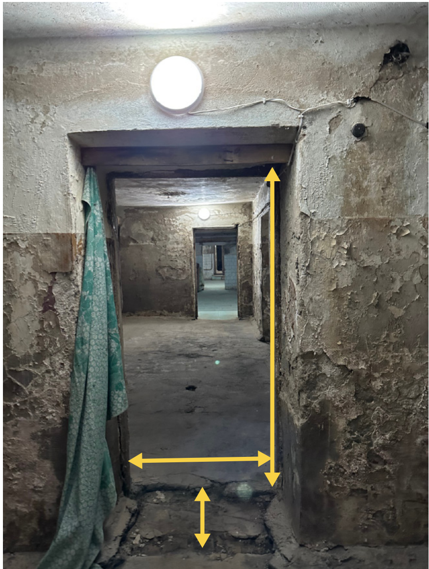
Doorway leading into a corridor. The plaster on the walls is worn out and flaky, and the concrete floor is damaged. Above the doorway there is a fixture and on its left, there is a green blanket acting as an improvised curtain. The image also contains yellow double arrows showing the dimensions that need to be measured: doorway height, depth and width.
